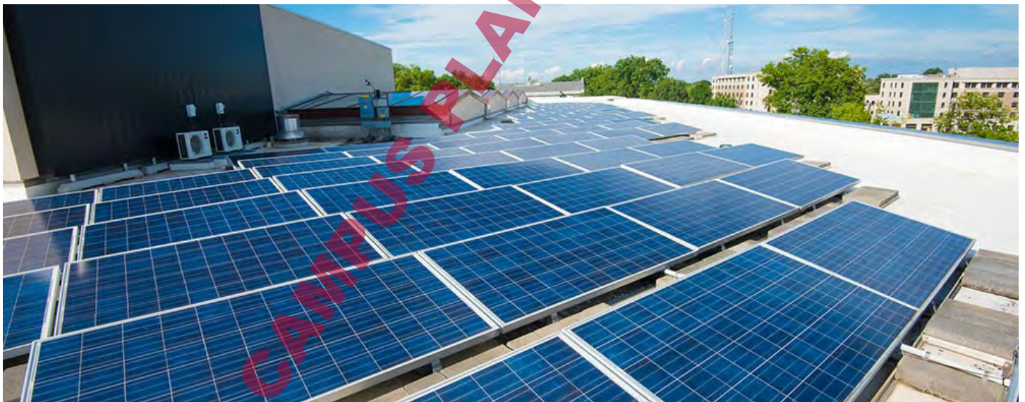
Rooftop solar panels at AU
